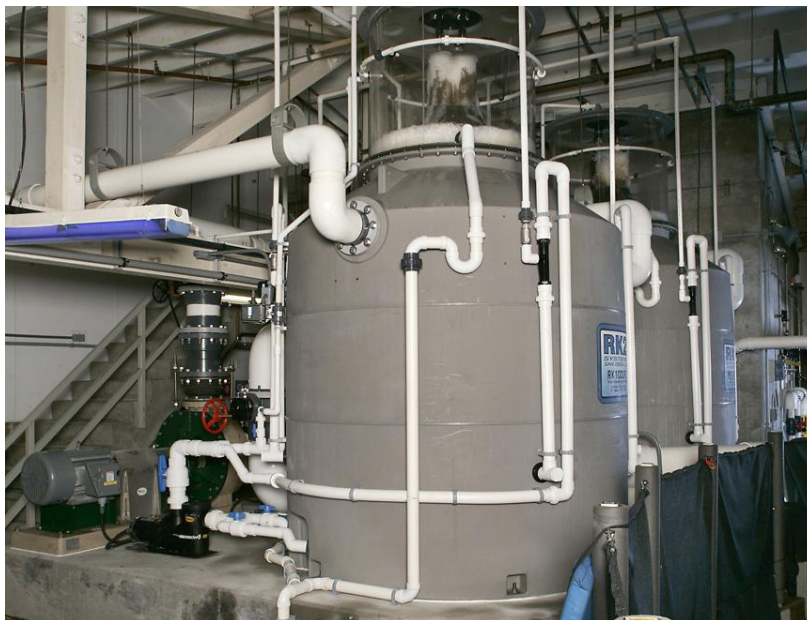
Figure 11. A picture of the two RK1000PE foam fractionators that were added to the OBW Exhibit life system in September 2004.
