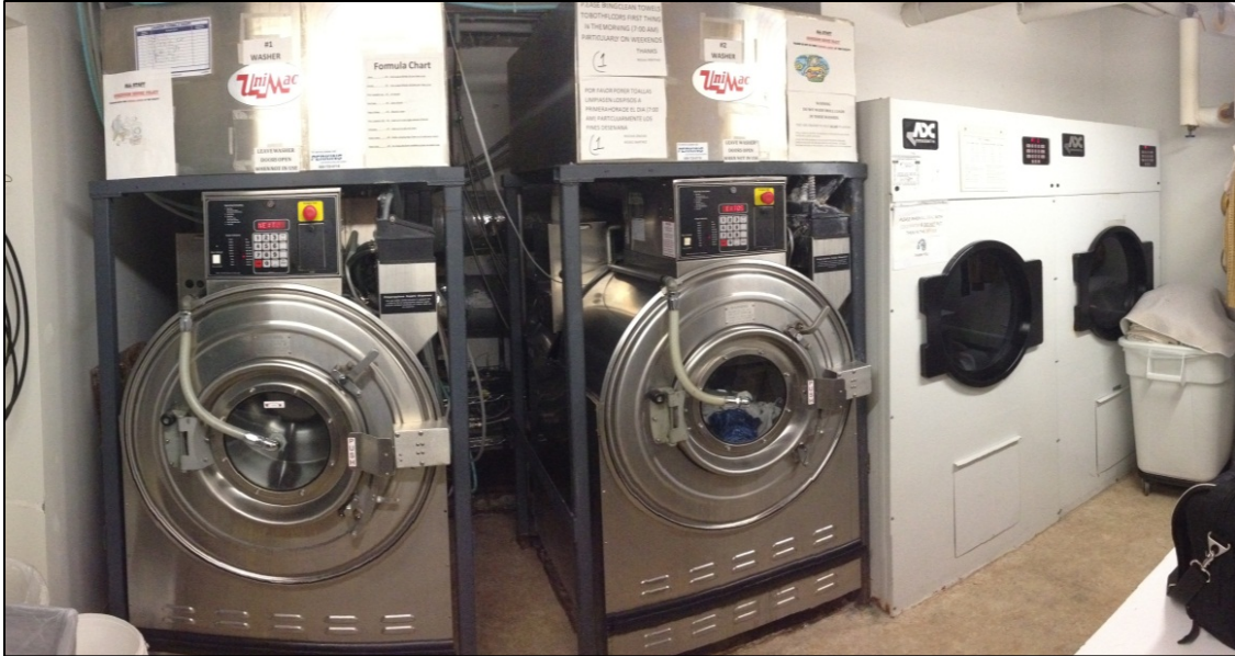
Figure 5. Rogerson House Laundry Equipment (Photo: Navigant)
