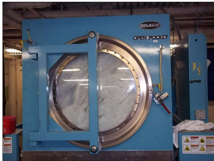
Figure 2. 250-pound Braun washer at the Charleston Place Hotel (Photo: Texchine, Inc.)
