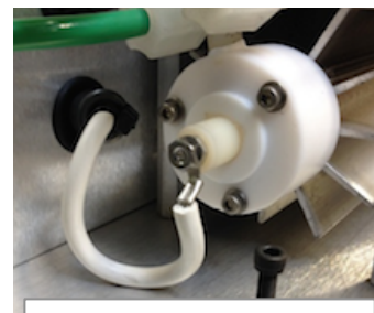
Bad - High voltage wire contacting metal
